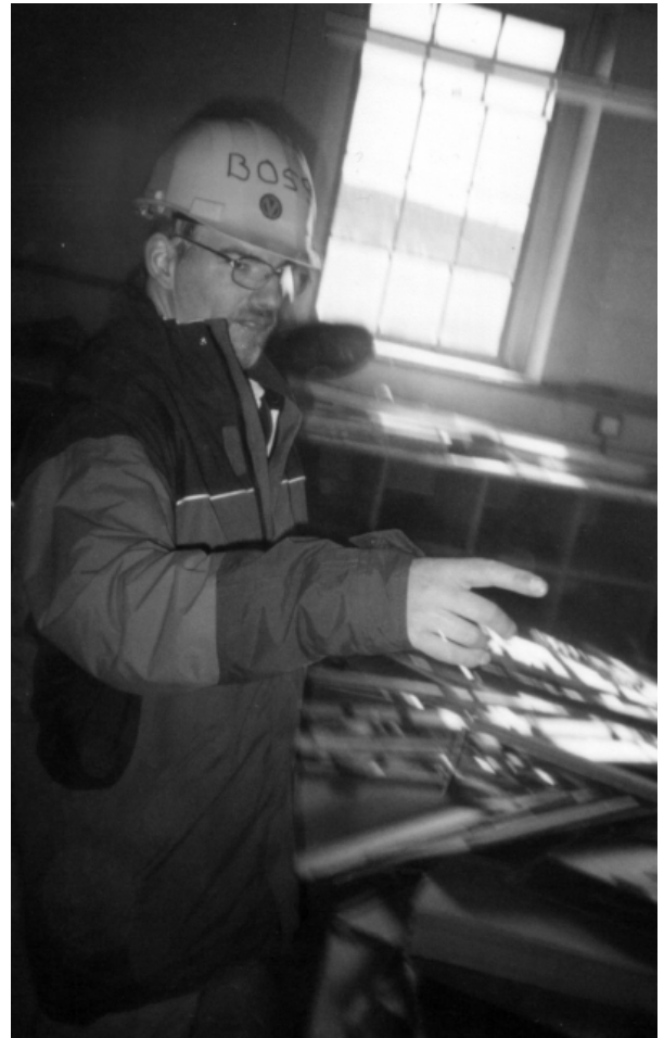
Client involvement: Simon Nunn takes charge of the refurbishment of the new offices
